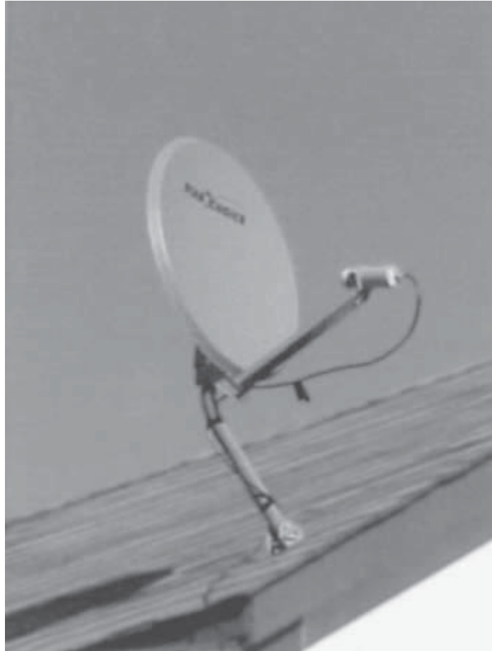
Figure 16.6 A typical DBS antenna installation.
